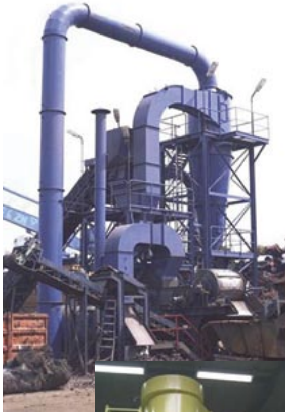
Cyclone erected with a shredder installation for the separation of 14 m 3 recycling product per hour.
