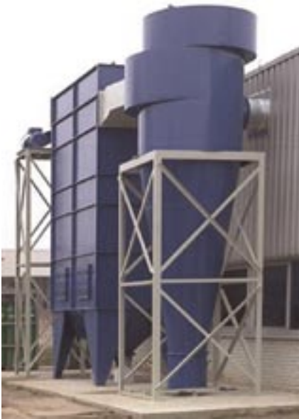
Cyclone erected with a Cobra-Jet bag filter for the separation of carbon fibre.
