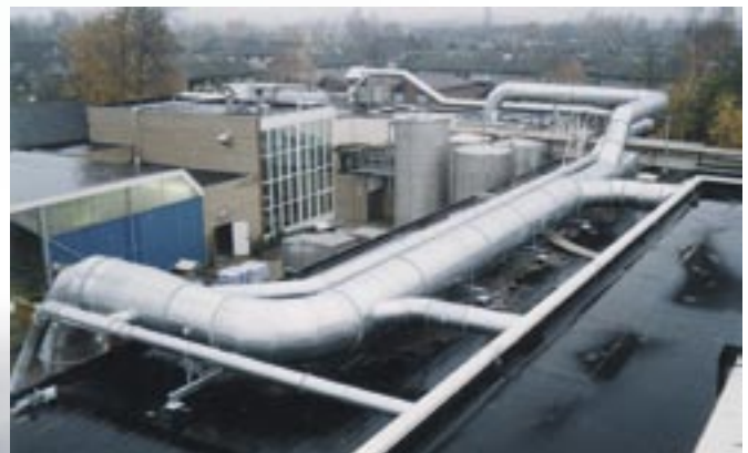
Flavour extraction in a slaughterhouse capacity: 60,000 m 3 /h
