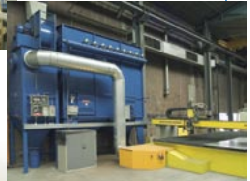
Cartridge filter type 20/21 erected behind a plasma cutting machine with a pre-separator and spark catcher. Capacity: 8,500 m 3 /h
