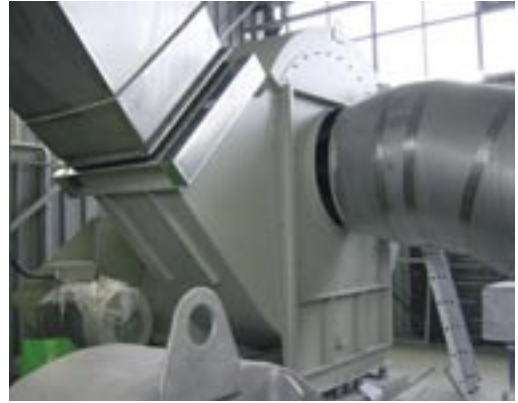
Fan type MH 45, capacity: 120,000 m 3 /h. Application exhausting behind milkpowder dryer.
