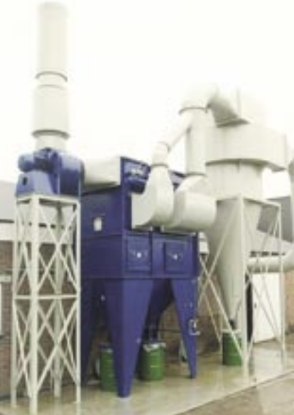
Pre-separating cyclone in metallization exhaust with cartridge filter type 26/21. Capacity: 15,000 m 3 /h.
